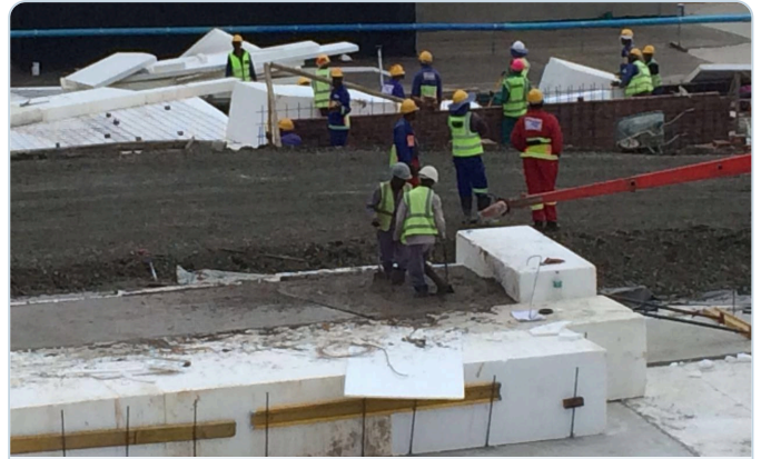
Placement — blocks positioned over the reinforced base and worked into the fill by hand.
