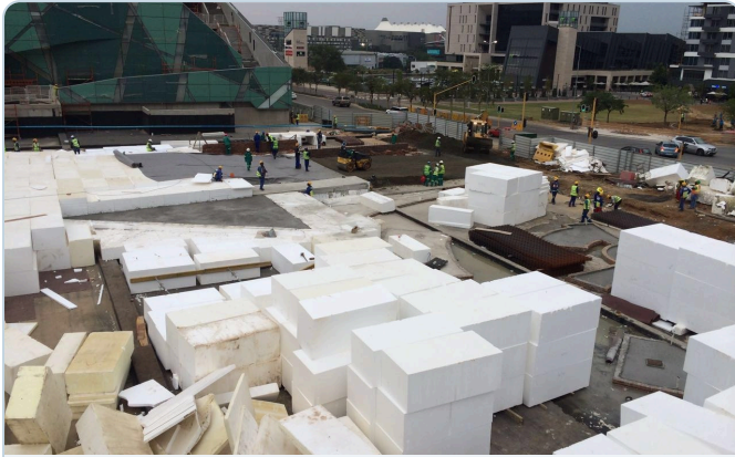
Delivered & stacked — blocks set out on site; light enough to place without heavy lifting plant.
