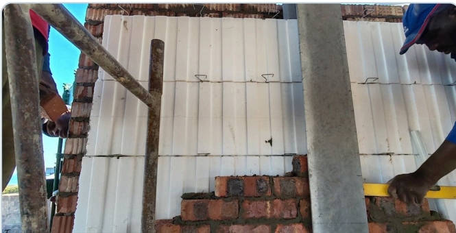
Cavity wall build — full-height fluted PolyKey EPS boards and wall ties built into a face-brick wall.
