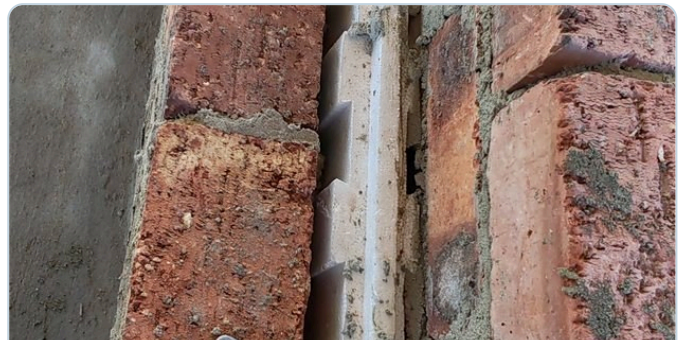
Cavity detail — keyed board profile, wall ties and a loose sample seen from above the cavity.
