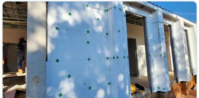
ETICS facade — Polyclad EPS backing boards mechanically fixed with anchor discs, ready for render.
