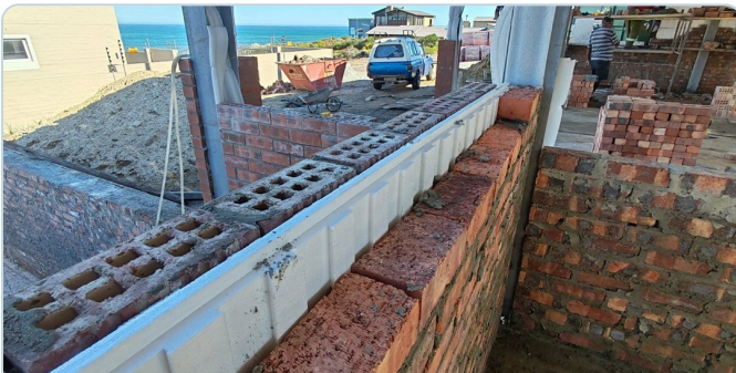
Coastal cavity wall — EPS boards between the leaves on a seaside residential site.
