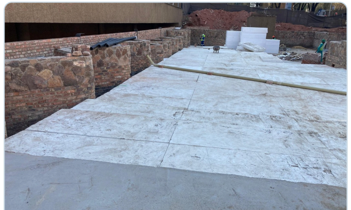
Completed works — RC slab cast over the fill, ready for the structure above.
