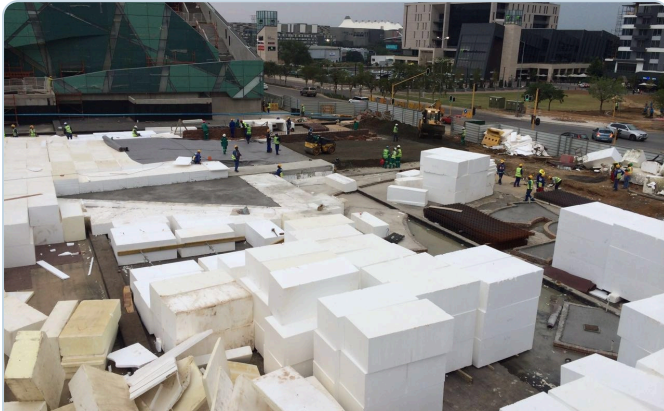
Delivered & stacked — blocks set out on site; light enough to place without heavy lifting plant.
