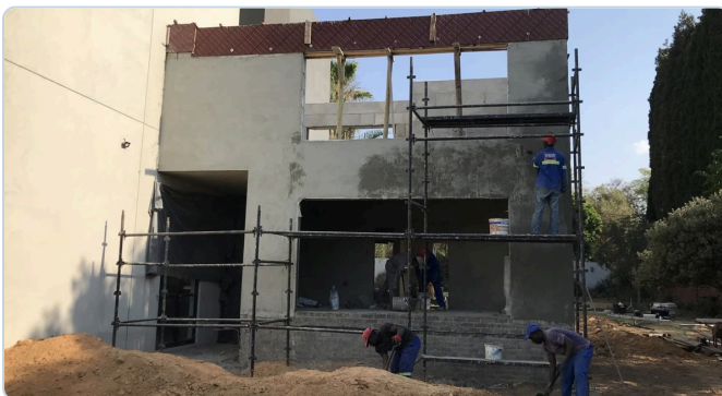
Render-skin stage — a double-storey building being plastered on scaffolding after the 14-day curing hold.
