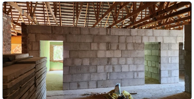
Internal LiteCore walls under conventional timber roof trusses — the block texture before the internal LiteCore Plast coat.
