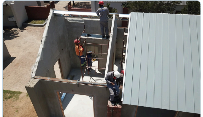
Wall plate to roof — lightweight steel trusses and roof panels installed over LiteCore walls.
