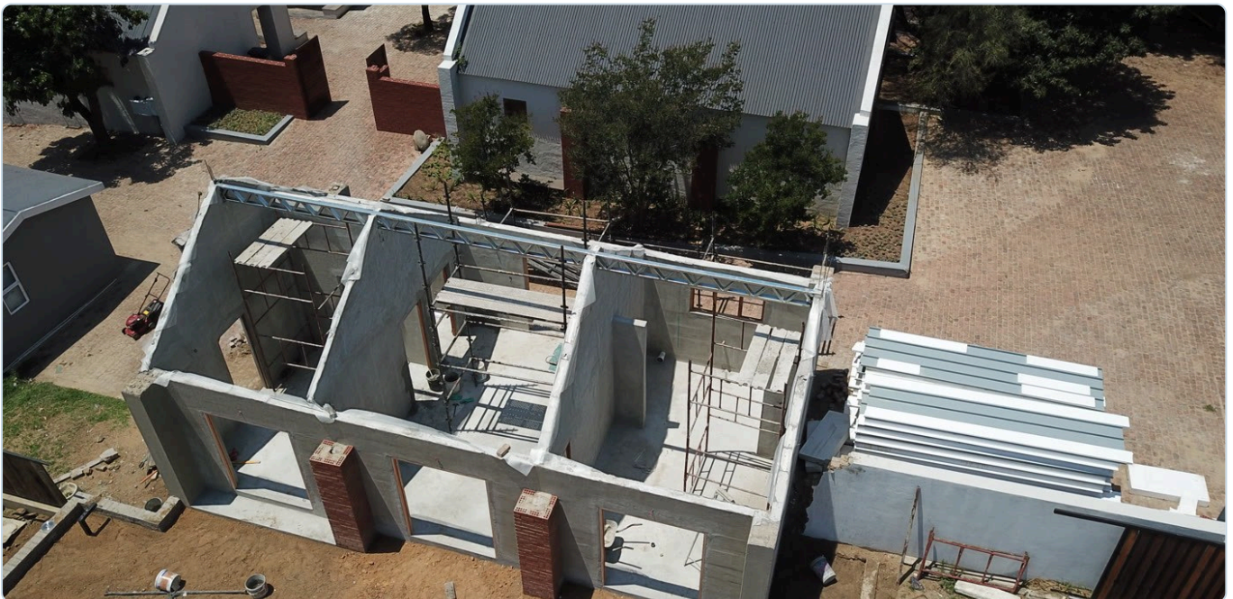
A LiteCore house at wall-plate stage — factory-cast blocks laid in thin-bed stretcher bond within an engineer-designed structure.
