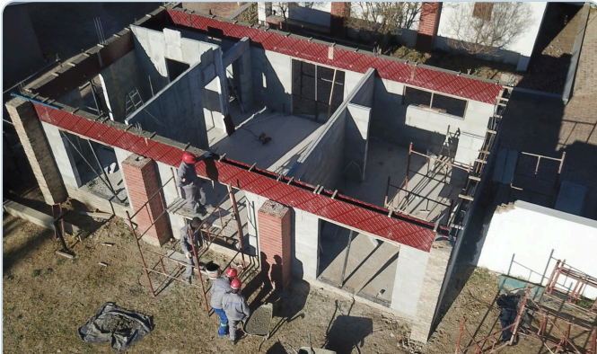
Ring beam & block laying — cast in-situ RC ring beams with columns carry the roof; LiteCore blocks infill between.
