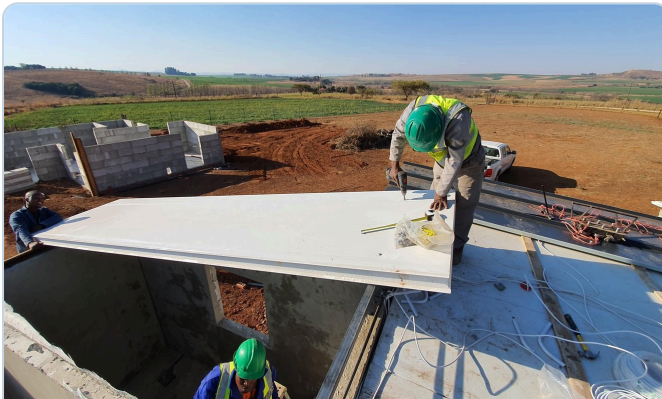
Installation — a white roof panel placed over blockwork; light enough to handle by crew.
