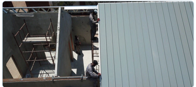
Standing-seam roof under installation — clips fixed, seams closed as the run advances.
