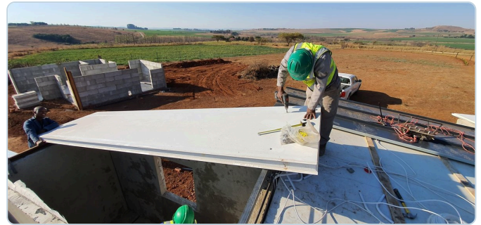
Panels handled on edge and worked into position on the fixed roof plane.
